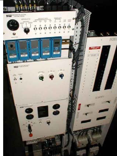
HVAC Control, Circuit Breakers, Generator Auto-Start, DC System Control, and Power Selection
